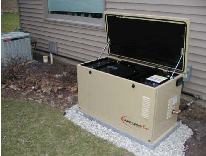
Fig. 14.2. A 7-kilowatt standby generator installed outside of a house, next to the air-conditioner. A 20-kilowatt cold fusion generator will be roughly this size. Photo by D. Kontac in product review on Amazon.com.
