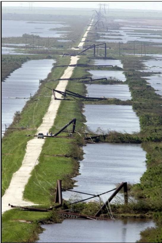
Fig. 14.1. Power lines damaged by a storm, Florida 2004. Power distribution lines are the Achilles heel of the power companies.
