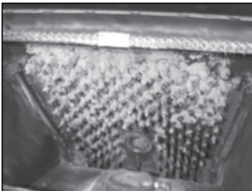
Figure 1 - Example of a dirty heat exchanger
