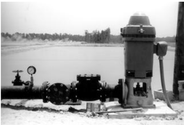
Figure 14. Large agricultural well with electric motor
