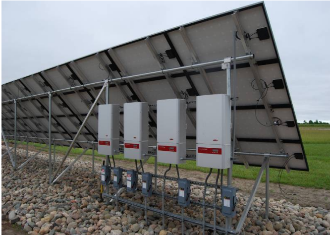
Figure 7: Fronius Inverters for power collection and performance monitoring
