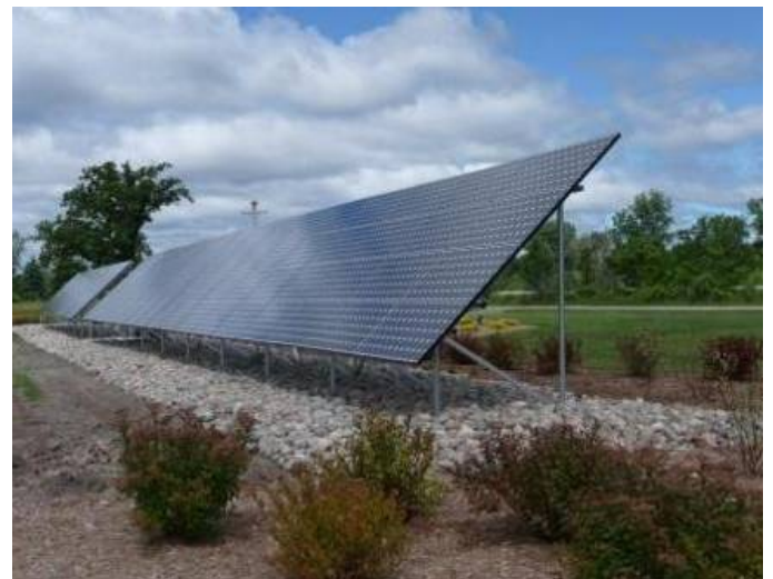
Figure 6: 30 Kw Array at Dow Corning Corporation, Auburn, Michigan, USA
