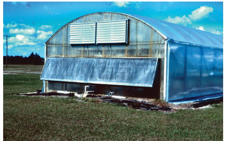
Figure 6. Cooling-pad endwall with open area for evaporative pad (in this photo, covered with motorized shutter) and 2 openings for motorized shutters, above cooling pad.
