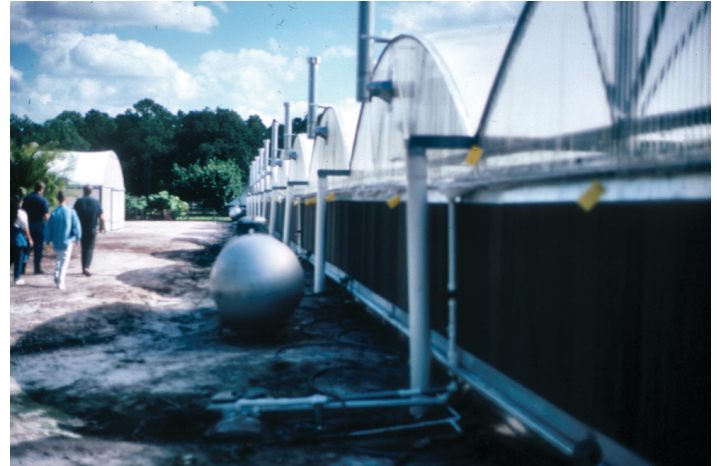
Figure 8. Evaporative cooling pad with underground water return system.
