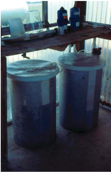
Figure 10. Entrance air-lock porch provides space for fertilizer stock tanks.
